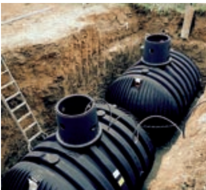
Depuradora en gasolinera. oneAdvanced 60 HE
